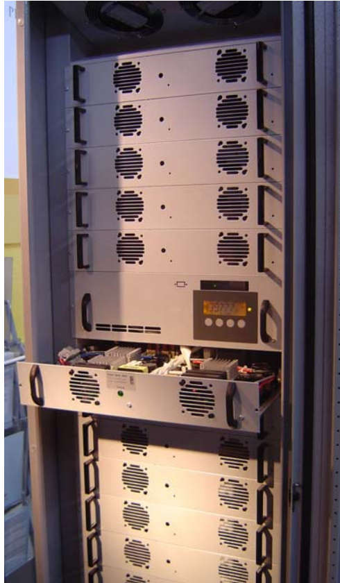
Rack with several higher-power inverters working in parallel
